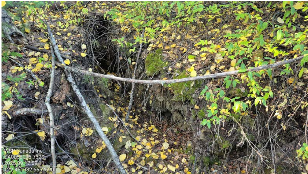
Photo 21 – vegetation mat tears, possibly indicative of ground movement.
