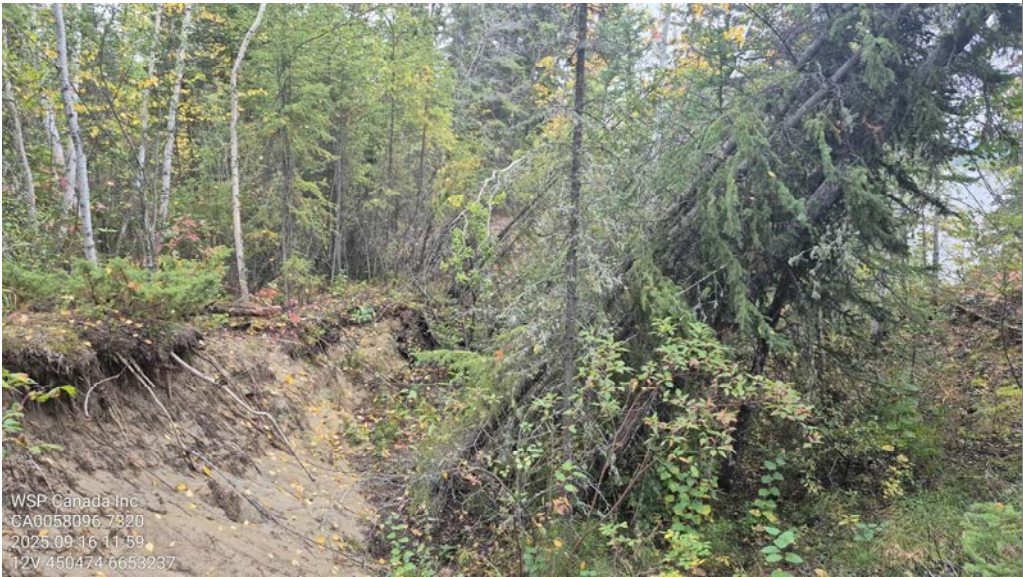
Photo 12 – scarp with exposed soil and mature tilted trees
