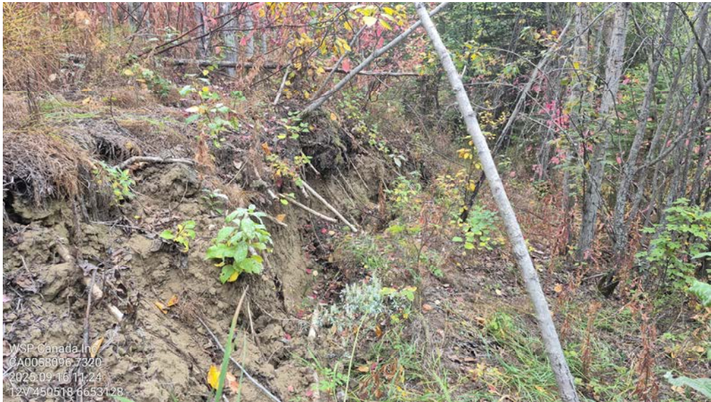
Photo 8 – area of fresh ground movement, torn vegetation mat and tilting trees/brush
