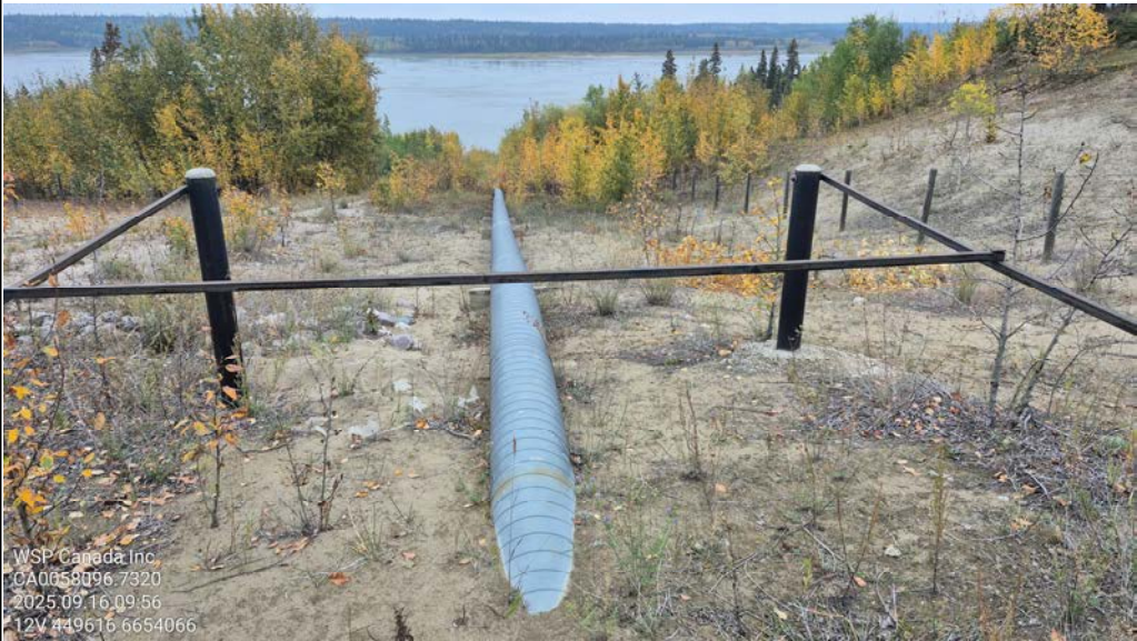
Photo 4 – water outfall pipeline near crest of slope, showing exposed sandy soil
