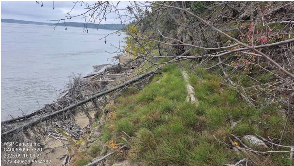
Photo 2 – erosion along toe of the slope
