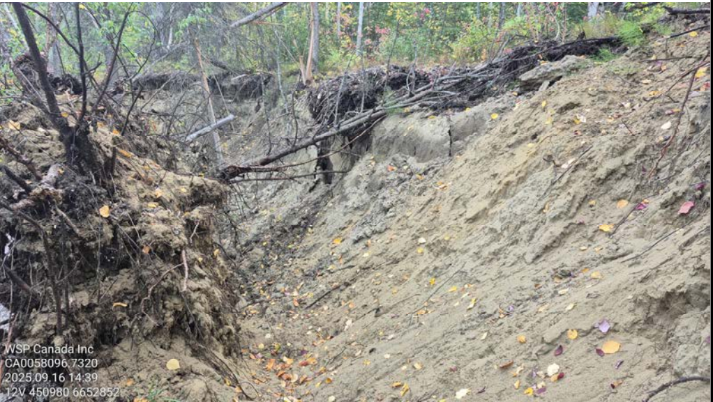
Photo 18 – scarp with exposed soil, exposed tree roots, split and damaged trees
