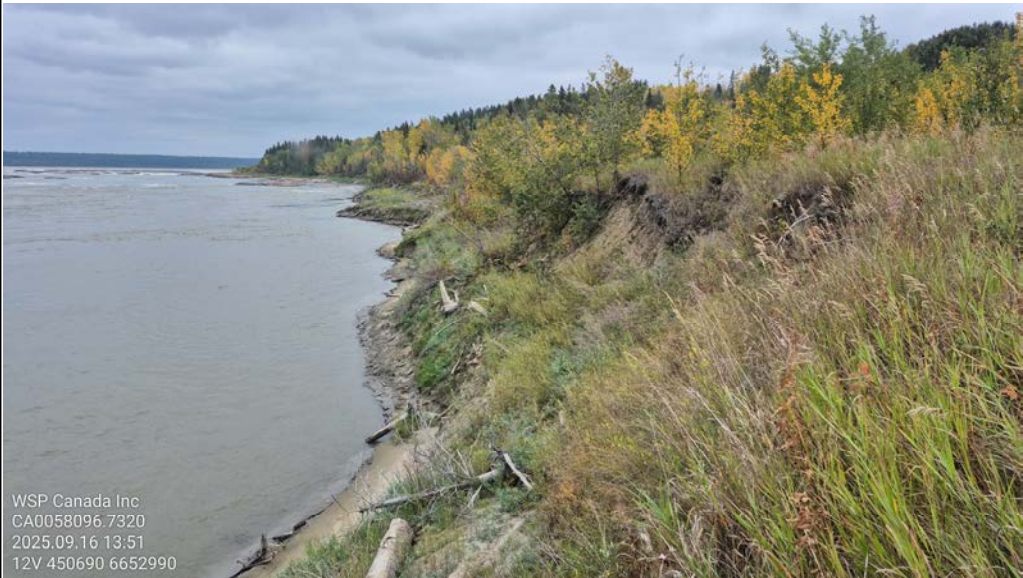
Photo 13 – scarps and benched topography along river showing erosion
