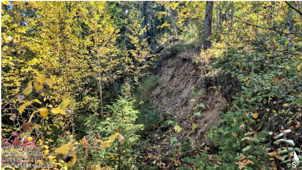
Photo 29 – headscarp with exposed soil
