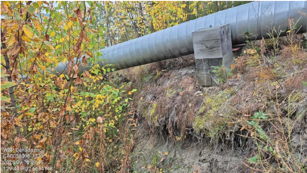
Photo 3 – scarp crossing under the water outfall line, and likely impacting support pad
